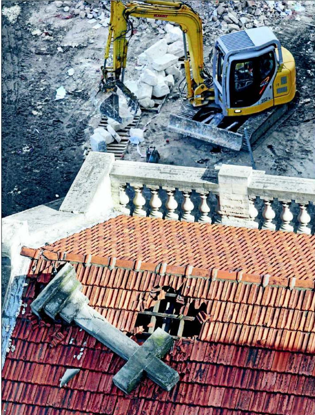
Victim: Work under way at the quake-damaged Cathedral of the Blessed Sacrament in Barbadoes St, Christchurch.
