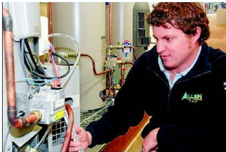
LIVE WIRES: Thanks to industry donations of fully wired and piped appliances, apprentices such as Chris Downey get to practice their diagnosis and repair skills in 'live' settings.
